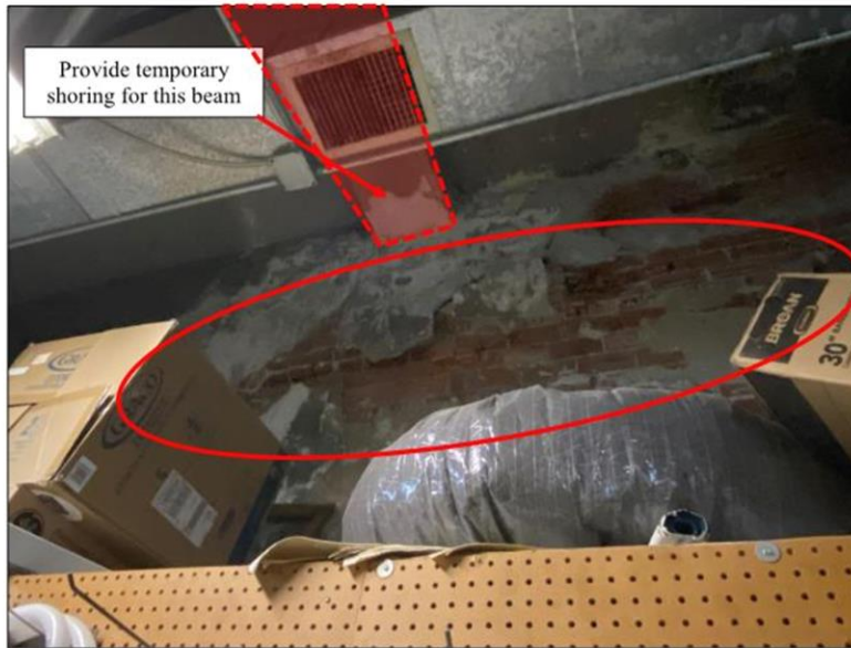
Photo 1 – Damaged Brick & Beam to Support
