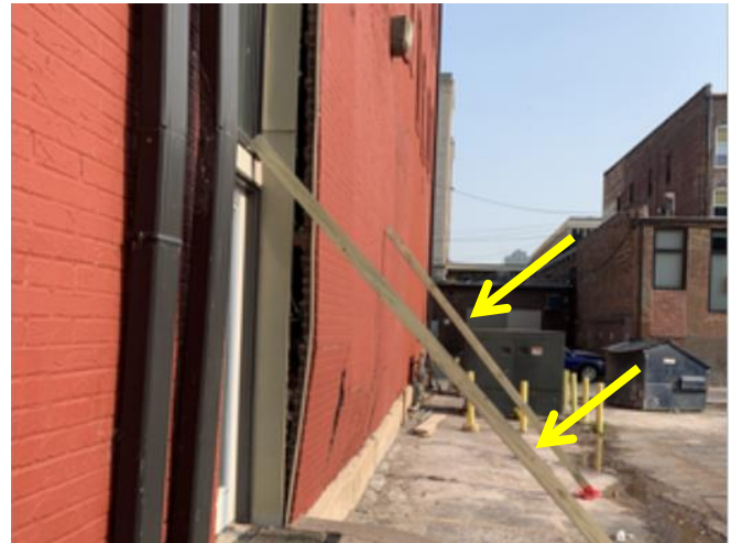
Photograph indicates area of bowing brick south of doorway. Note “shores” in place that do not appear to conform with SSE’s design.
