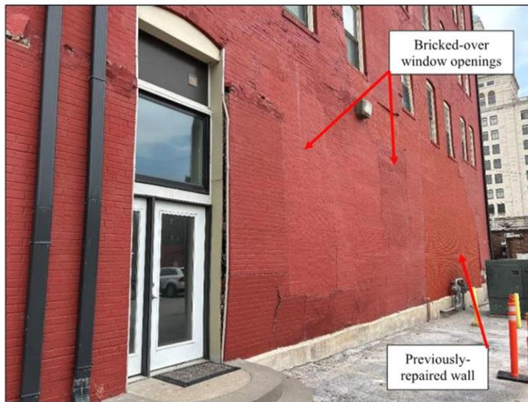
Photo 1 – Clay Brick Façade pulling away from Substrate
