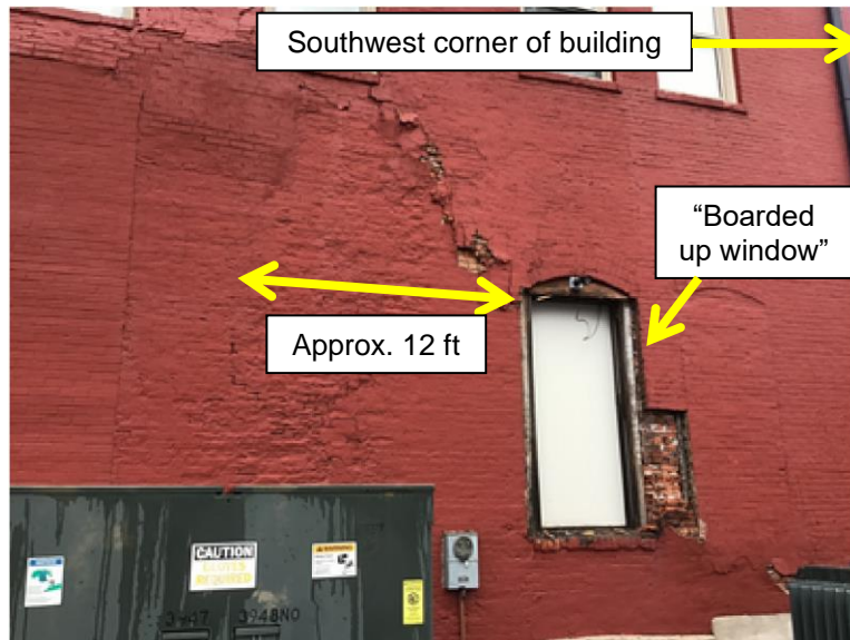
Fig. 35. View of assumed area of specified repair by SSE’s February 8, 2023 letter (Ref. City Report Task ID: 23-6454). Annotation by WBG and SEI.
