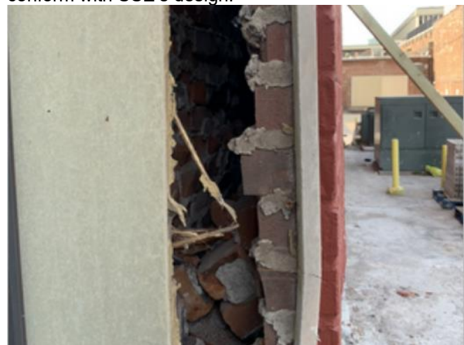
Detail view of bowing brick at south jamb of doorway. Note bricks accumulated in gap between wythes.
