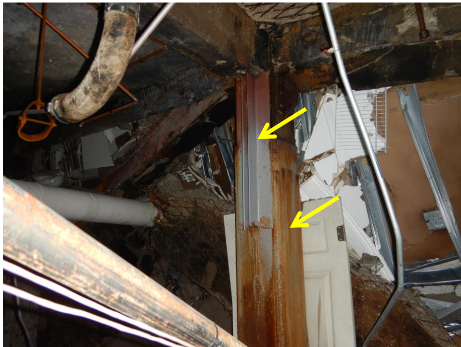
Photograph 34: Image and annotation by WBG/SEI of basement column. Note cover plates and steel angle beam seat reinforcement.
