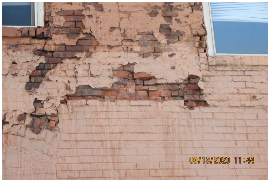
Photograph 4: August 2020 image of west elevation from City report. Note open mortar joints, spalling brick faces, and other masonry distress.
