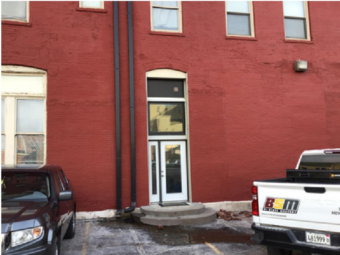
Fig. 31. Image of the west elevation adjacent to Unit 105 door taken on November 1, 2021 (Ref: City Report, Task ID: 21-64101).
