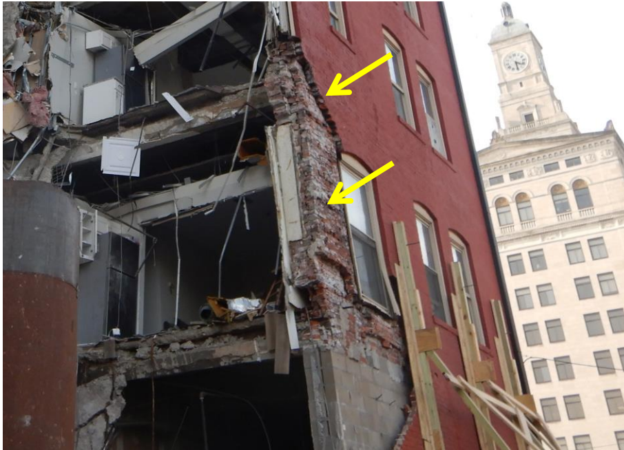
Photograph 19: Post-collapse view at wall cross section. Note outer 2 wythes of brick masonry not bearing on CMU replacement wall.
