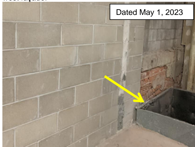
Photograph indicates area of replaced CMU from inside. Note mechanical opening in floor.
