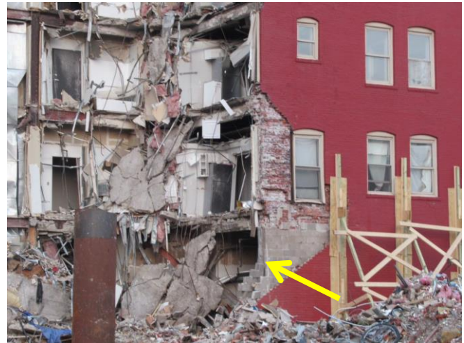
Fig. 21. Photograph of the southern extent of the collapsed portion of the Building taken June 4, 2023. Arrow indicates construction joint of new CMU wall construction.
