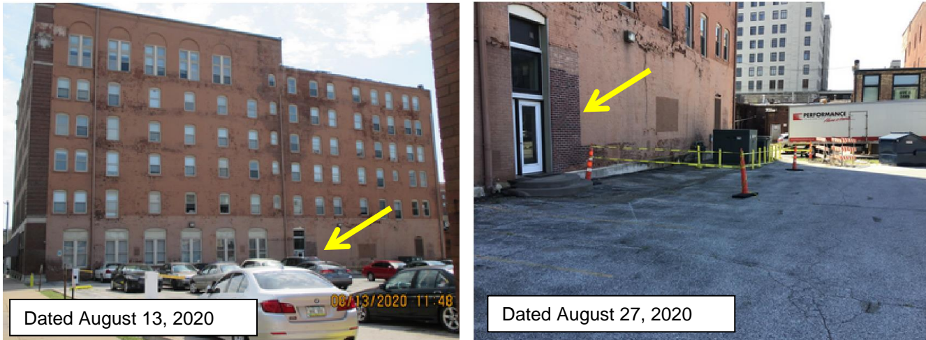
Fig. 26. Images of the west elevation (Ref: City Reinspection Reports, Task ID: 20-7839 and 20-58268). Yellow arrow points to area of apparent previous repair.
