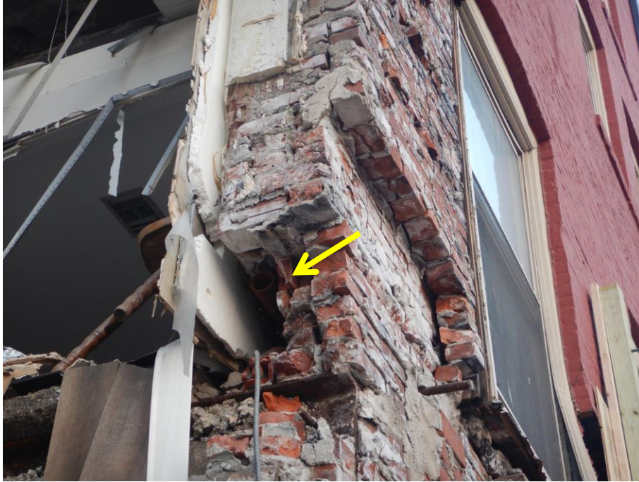
Photograph 25: Post-collapse image of cross section of wall. Note reduced wall thickness at location of plumbing embedded within wall at Pier G.
