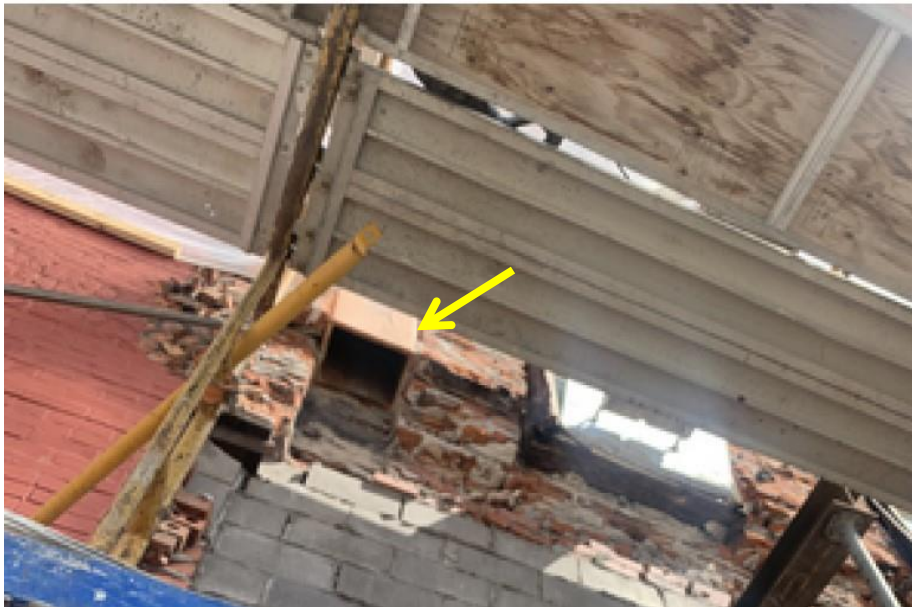
Photograph 26: Image from City file 23-9778 exhibiting April 2023 repair work. Note large vertical chase embedded within wall at Pier F.
