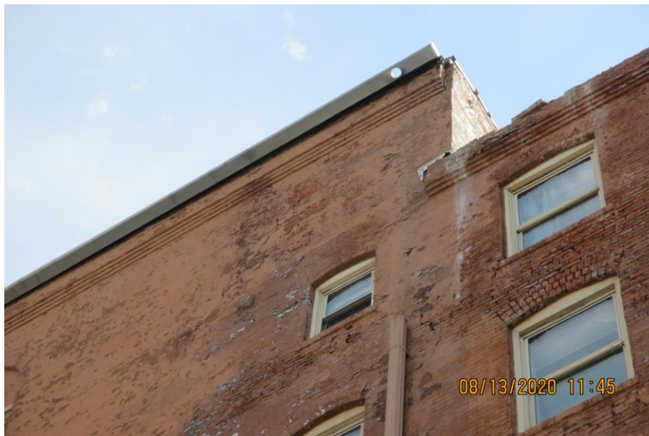
Photograph 2: August 2020 image of west elevation from City report. Note open mortar joints and masonry distress.
