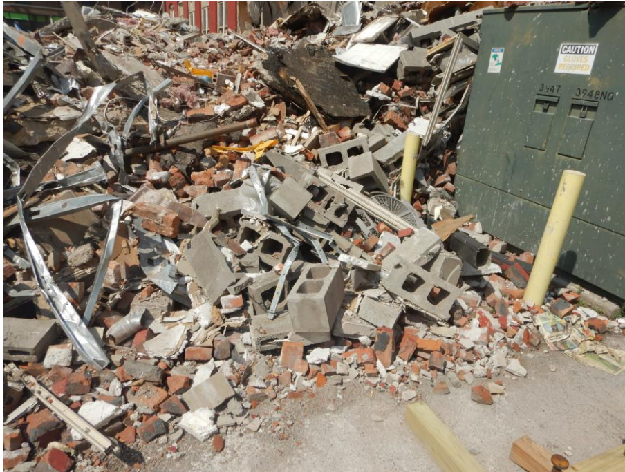
Photograph 17: Post-collapse photo of west elevation wall debris. Note lack of reinforcing steel or grouted cells in CMU wall component debris
