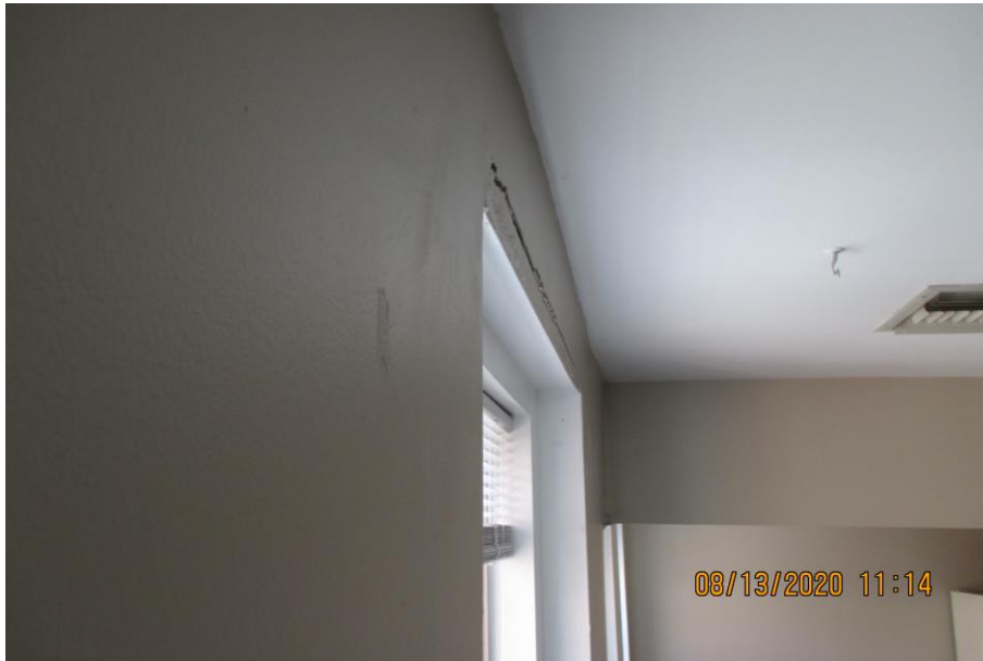
Photograph 29: Image from City file 20-7839. Note indications of water infiltration and distress at ceiling and window head.
