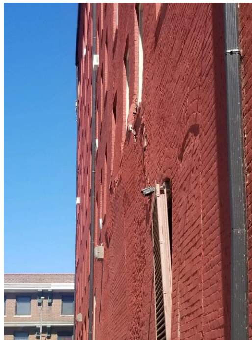
Photograph 10: February 2023 image from City file 23-6454. Note displaced masonry and louvers.
