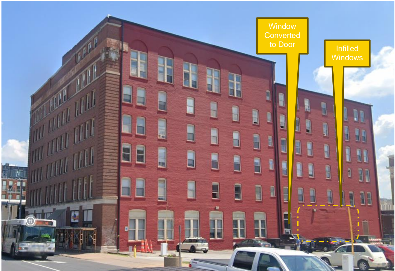
Fig. 4. Overall view of the west elevation of the Building (Ref. Google Streetview, dated June 2021). Annotation by WBG/SEI.
