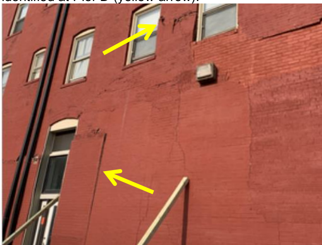
Overall view of portion of west elevation south of door. Note numerous areas of deterioration to wall.
