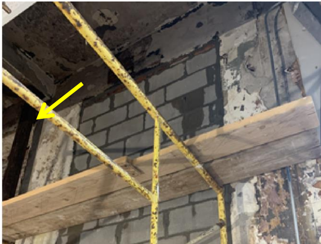
Photograph indicates inside of building with CMU installed inside window opening. Note shore previously identified at Pier D (yellow arrow).
