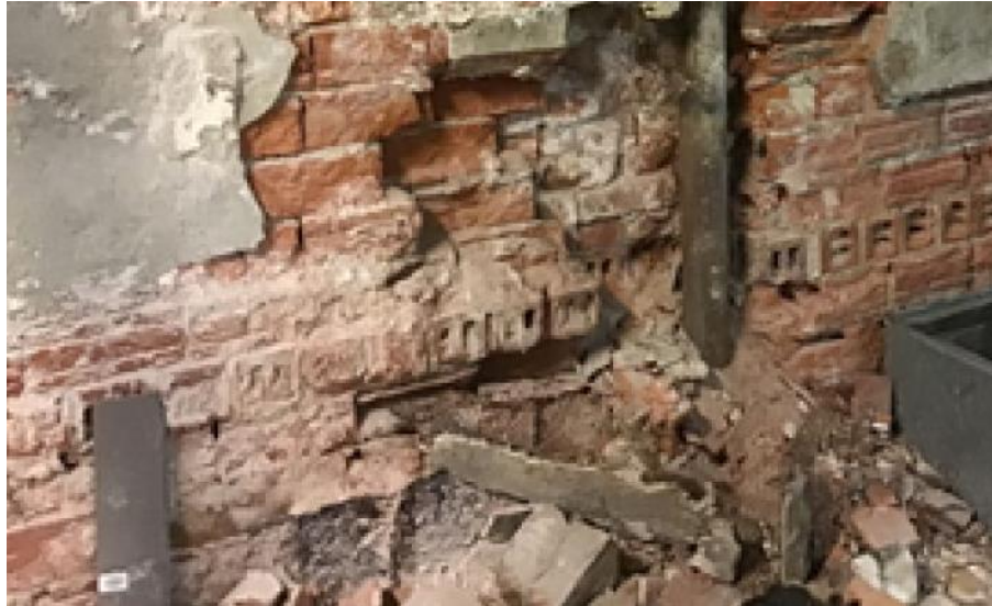
Photograph 11: February 2023 image from City file 23-6454. Note distress and damage at interior masonry.
