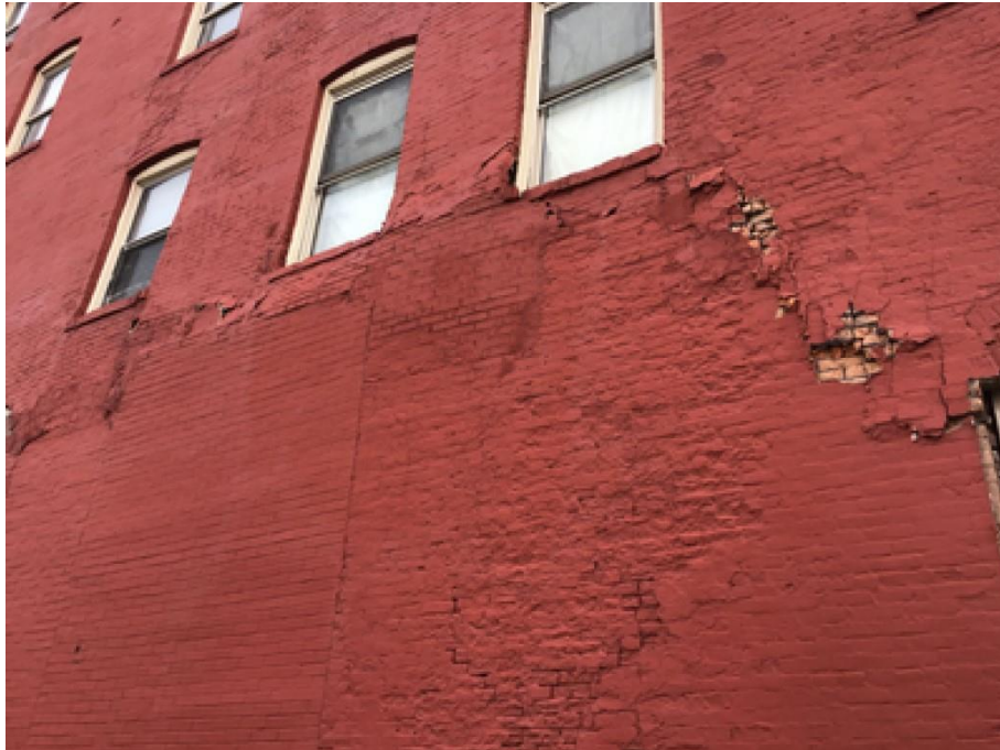
Photograph 9: February 2023 image from City file 23-6454. Note shear cracks and displaced masonry.
