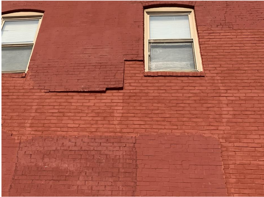
Photograph 27: Image from City file 23-30329. Note mis-aligned masonry at Pier E brick replacement locations.
