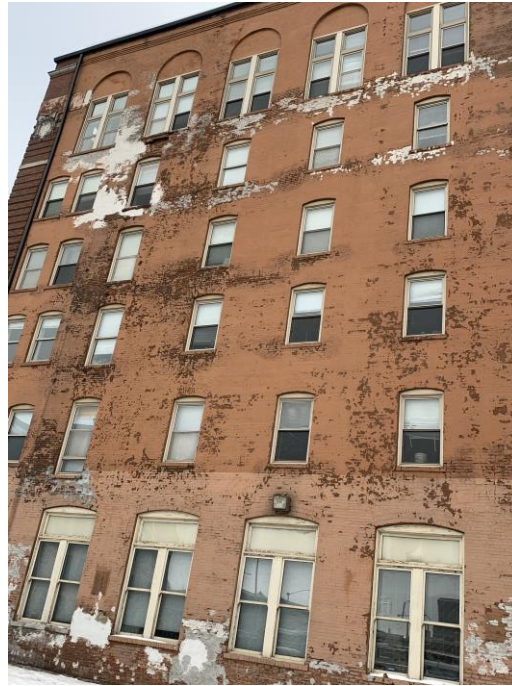
Photograph 5: 2021 image from City report. Note masonry deterioration throughout west elevation.
