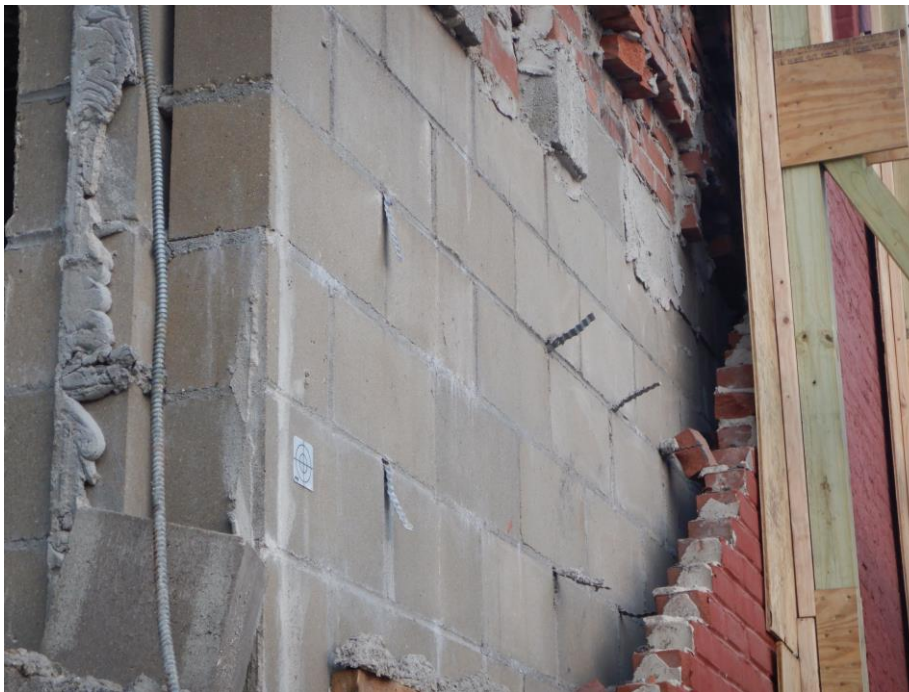
Photograph 20: Post-collapse image of CMU wall constructed in May 2023. Note corrugated brick ties not engaging outer wythe of brick masonry.
